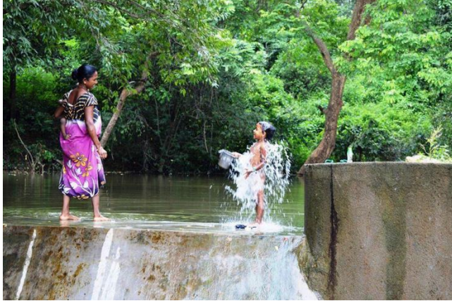
Fig. 4. A photograph of Water Harvesting structure and catchment forest in the background
