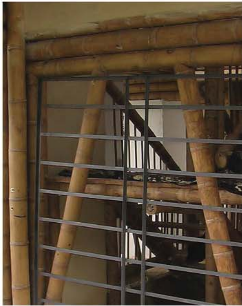
Incompatibility with building elements
